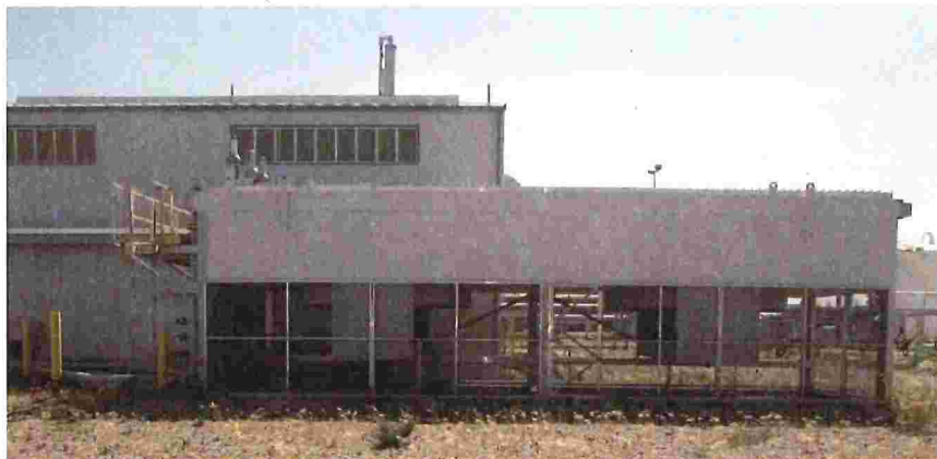
Sweet Gas Compressor Coolers E2209-10 A/B
