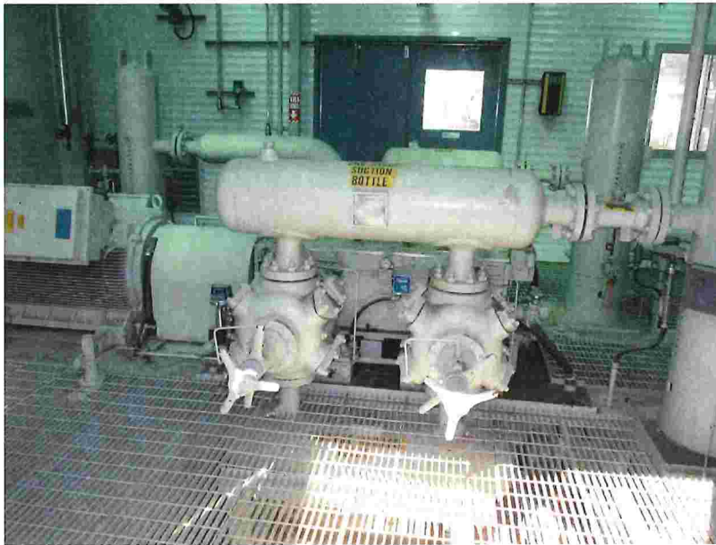
Recycle Compressor C-2705
