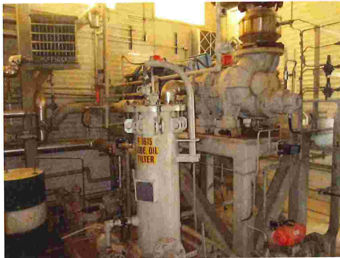
Refrigeration Compressor C-3660
