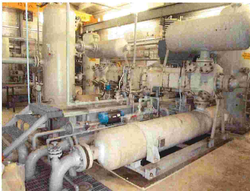
Sweet Gas Compressor C-2200 A
