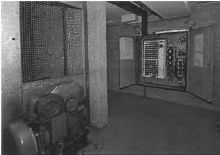
Elevator New Mechanical 3
