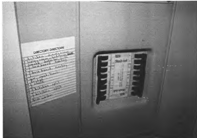
In- Suite Breaker
