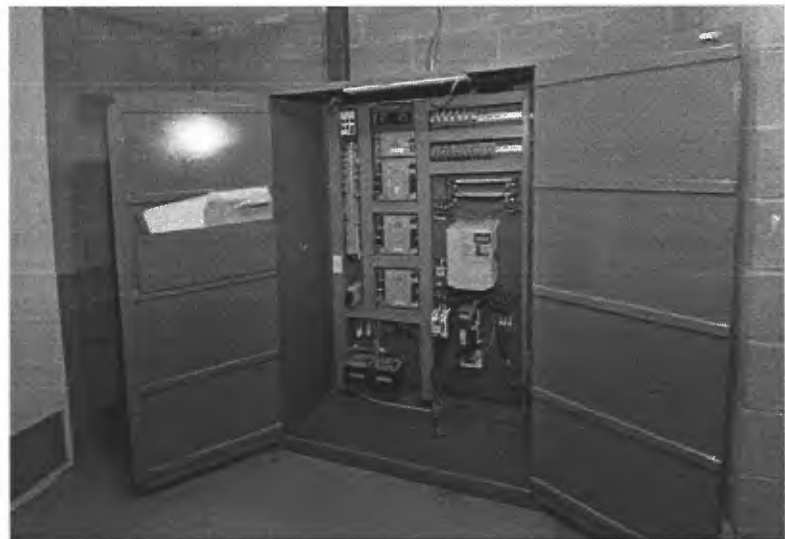
Elevator New Mechanical 2
