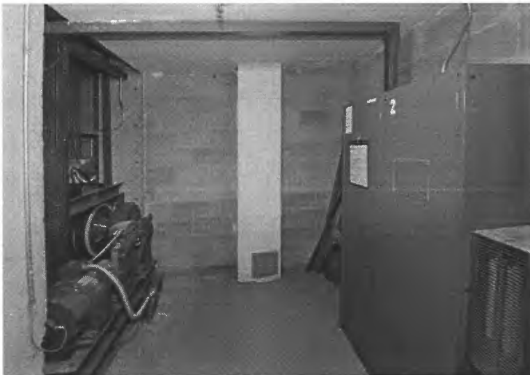
Elevator New Mechanical
