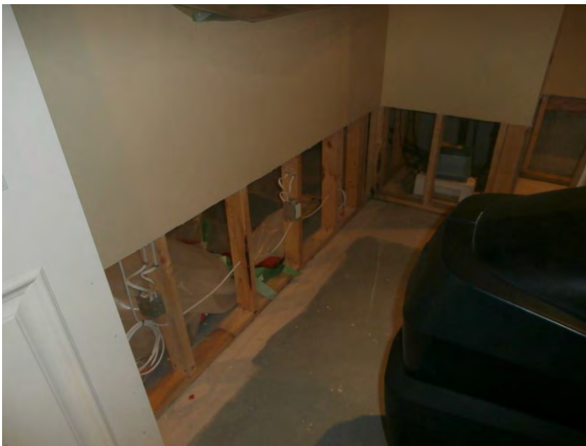
Basement Water damaged walls
