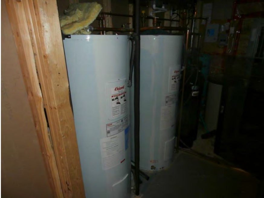
(2) Electric 80 Gallon Hot Water Tanks
