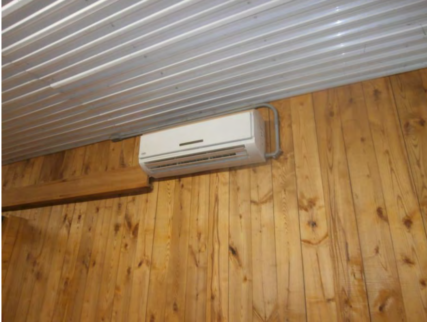
Wall Mounted HVAC
