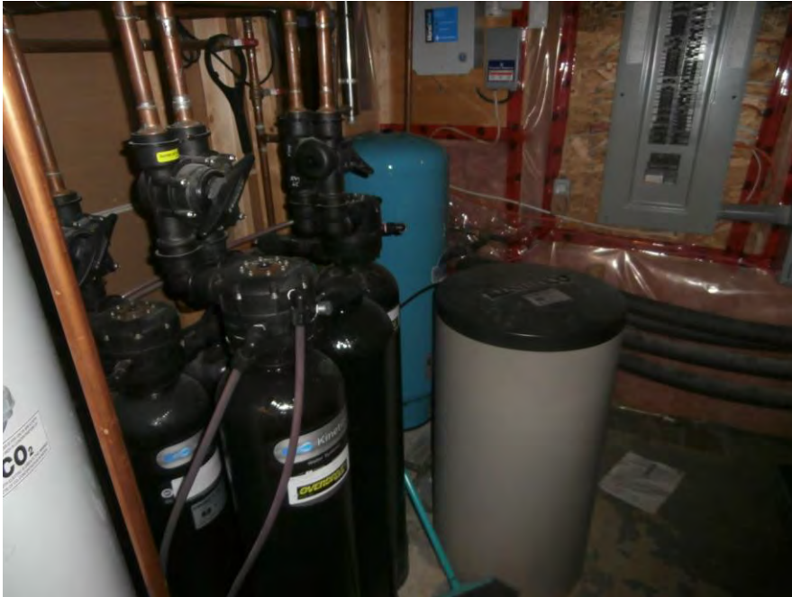
Water treatment System and Electrical 240 Volt 400 Amp System
