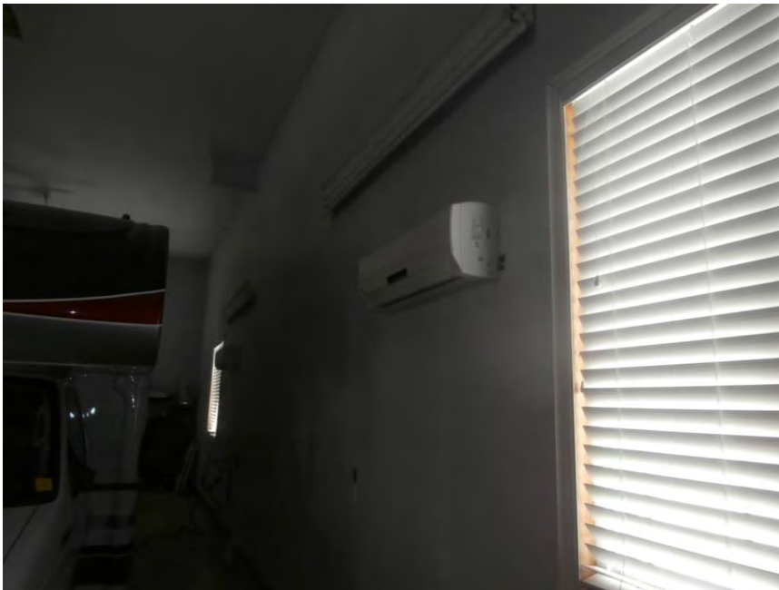
(2) Wall mounted HVAC units
