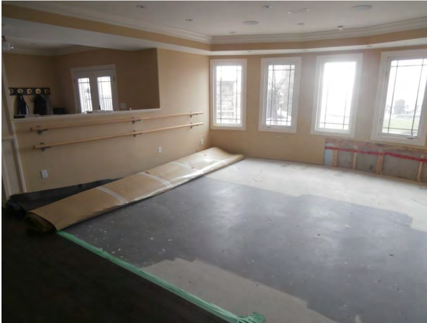
Basement Dance Studio and Water damaged floor
