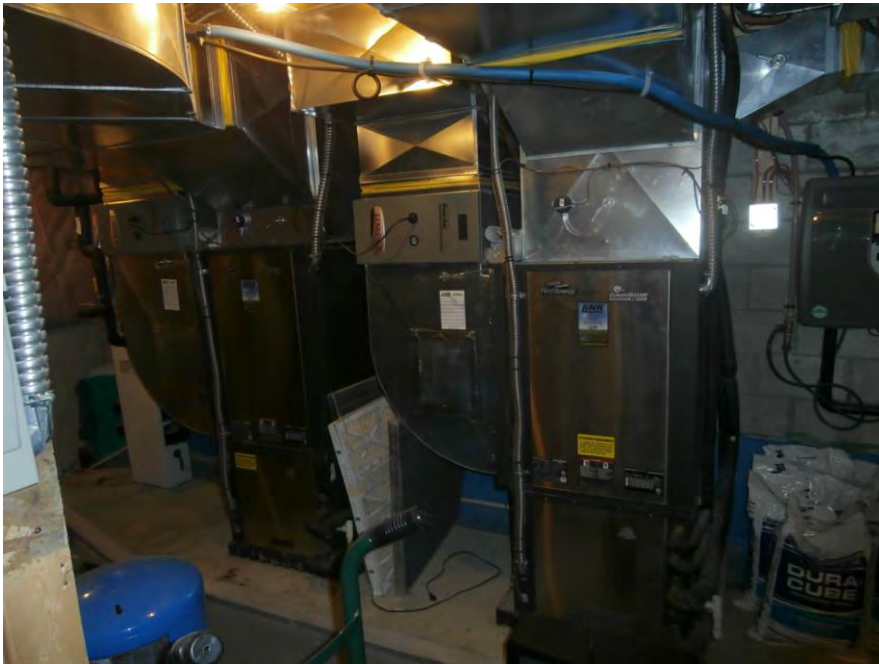
(2) Electric Forced Air Ground Source Furnaces
