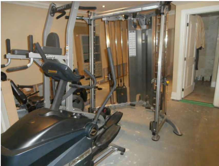
Basement Gym and Water damaged floor
